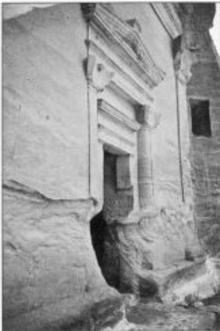
Figure 1 Rock-cut façade of a tomb at Petra, Jordan, showing severe salt damage along the base.
