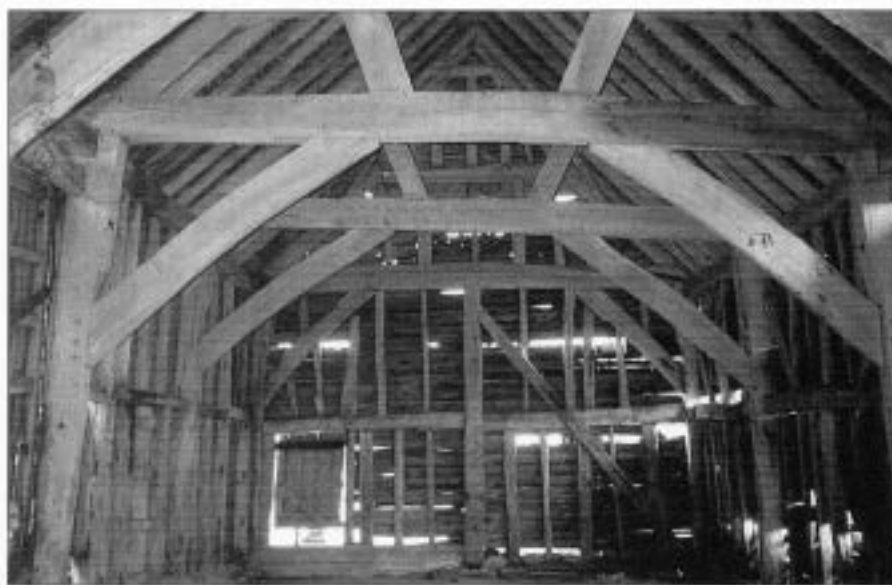
Figure 6 View of the east end of the south barn at Home Farm, Newdigate, Surrey. Dendrochronology revealed that this was built of timbers felled in the winter of AD 1608–9.
